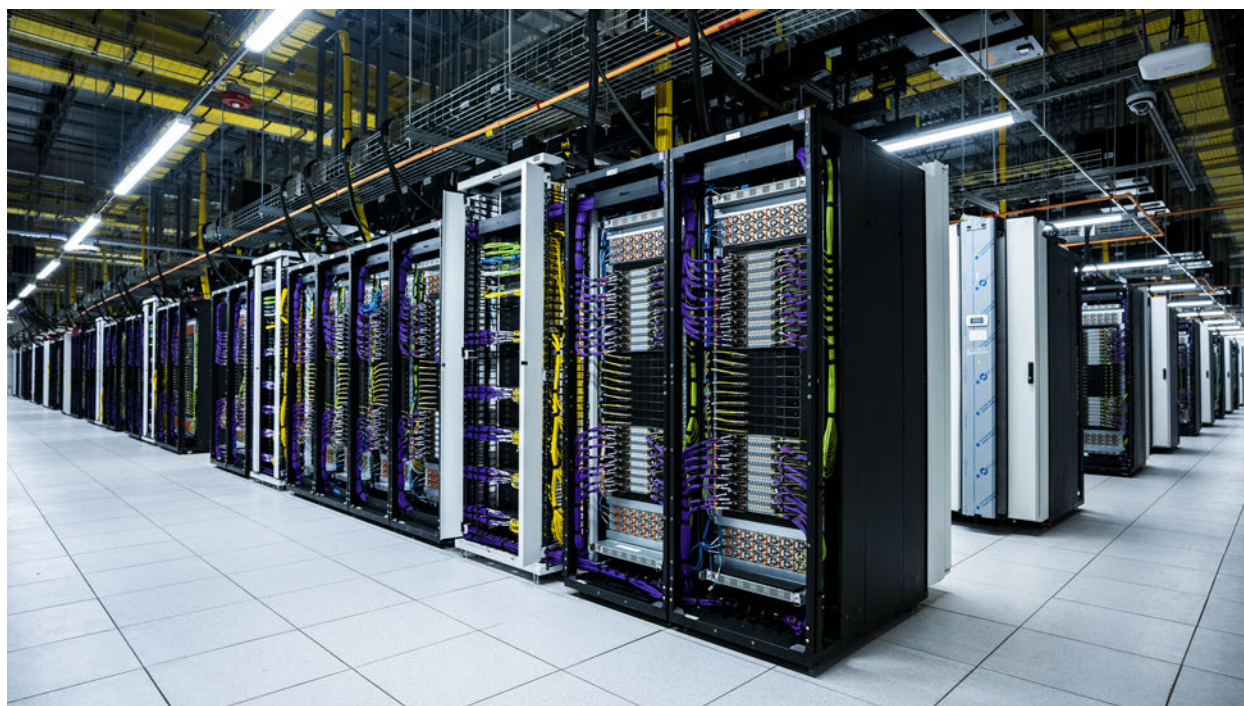
COLOSSUS II Facility in Memphis, Tennessee
